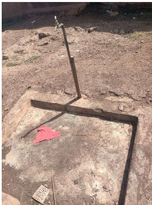
Tap mounted over drainage slab — limited hygiene and reliability without storage
