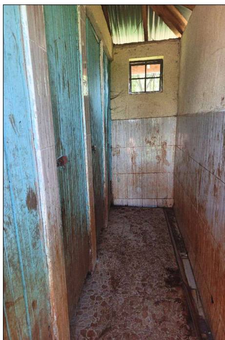
Interior corridor of a toilet block: worn surfaces and poor drainage
