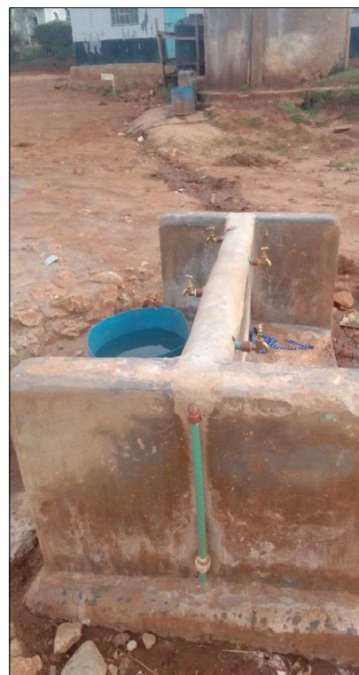
Communal handwashing station with multiple taps — durable structure with moderate accessibility
