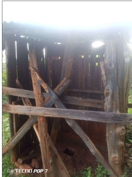
Figure 9: Severely damaged pit latrine made from unreinforced wooden poles — unsafe and unfit for learners
