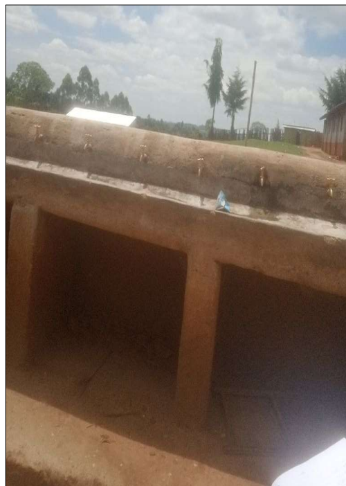
Large handwashing station with multiple taps — ideal but underutilized in many schools.
