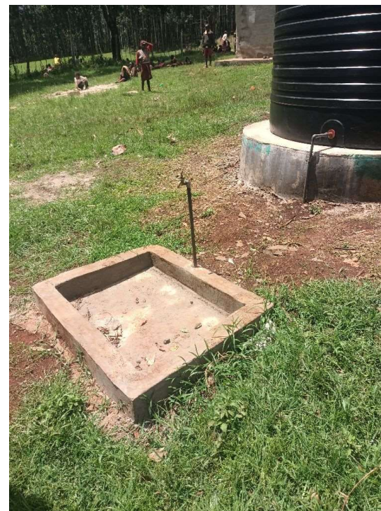
School tap connected to black tank, but lacking proper drainage
